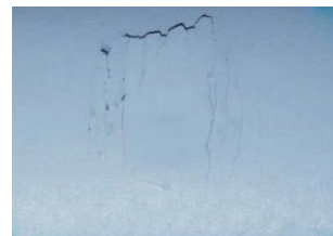
Fig. 1: FRP with painted surface and impact damage (8.5J)
